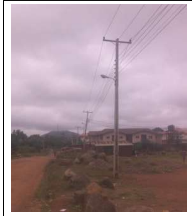
Plate 1: Electric Power Distribution Concrete Pole
